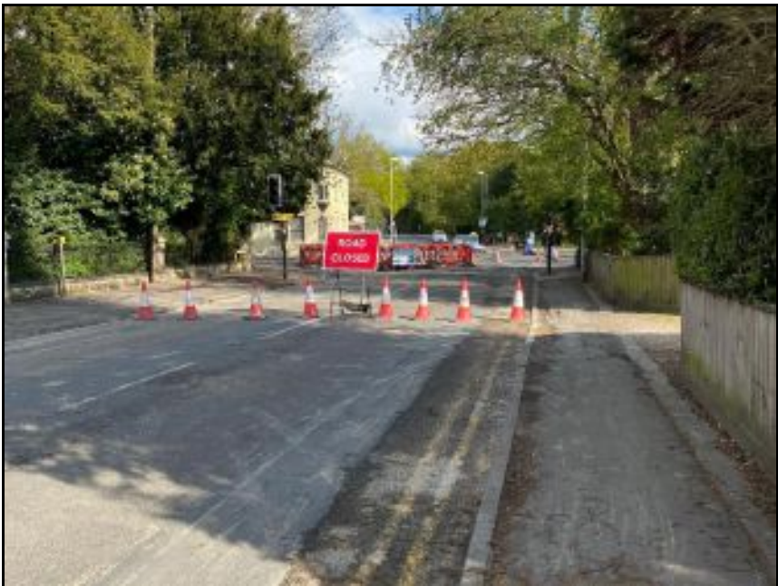
Burst water main leads to crossroads closure
